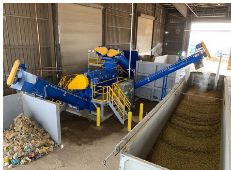
A new facility near Sacramento sorts and processes organic waste for use in anaerobic digesters that produce biomethane. | Republic Services
