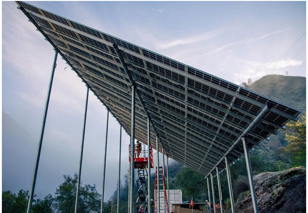
PG&E last year developed its first remote grid system to support Briceburg, Calif., an isolated community in Maricopa County that had previously lost service because of burned power lines. | BoxPower
