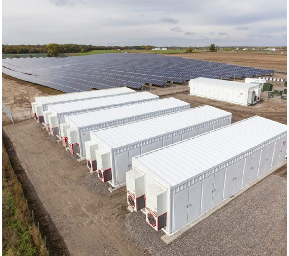
Connexus Energy solar and storage site in Minnesota | Connexus Energy
