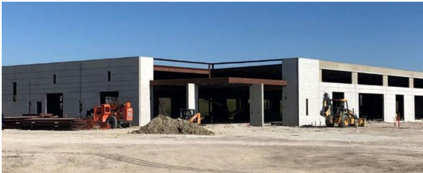
ERCOT's new headquarters building, under construction here in early 2021, is nearly ready for occupancy. | ERCOT
