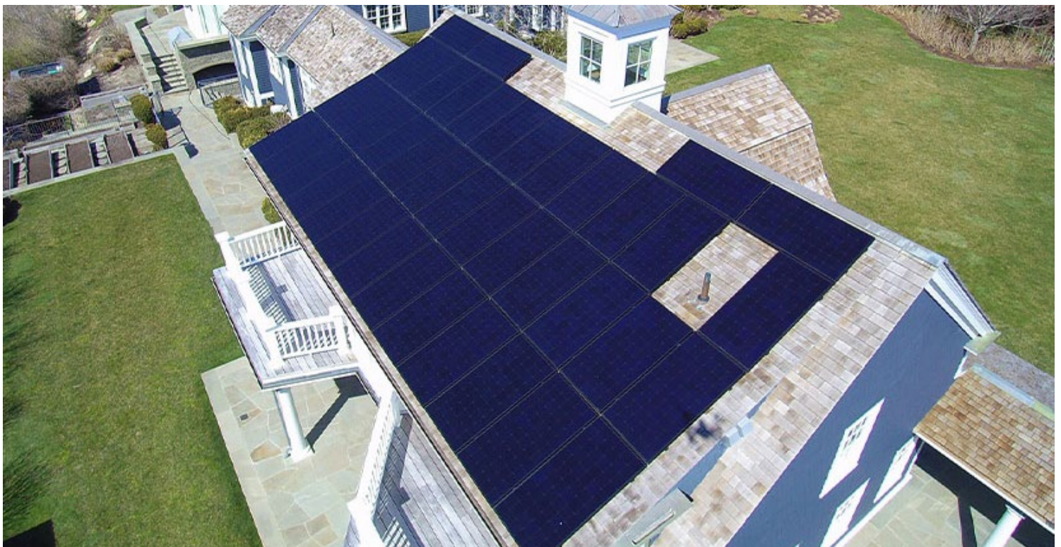
A solar installation on a house in Dennis, Mass. | DOE
