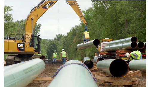
Construction of Consumer Energy's Saginaw Trail pipeline project in Michigan | Consumers Energy
