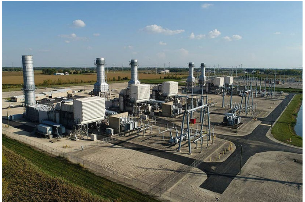
J-Power's Elwood Energy Center, a 1,350-MW natural gas turbine in Illinois | J-Power
