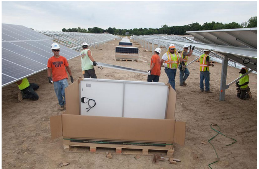
Construction of a DTE Energy solar farm in Michigan | J. Ranck Electric
