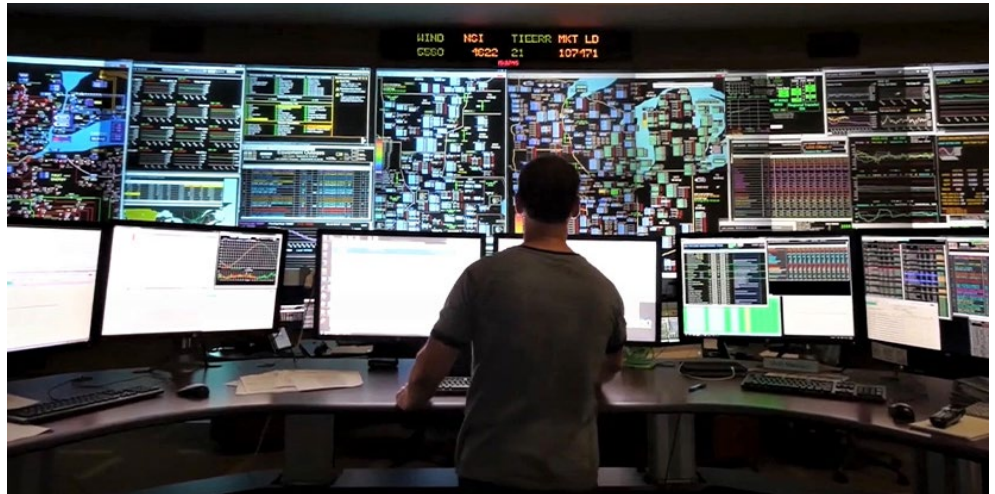
MISO control room | MISO
