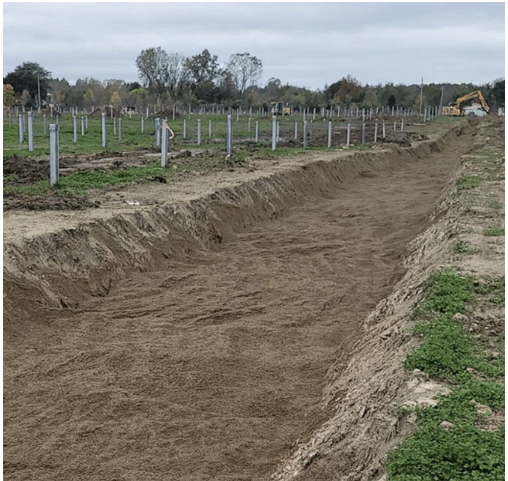
Construction of the Lyons Road Solar project in Michigan, a joint venture of Irradiant Partners and Pine Gate Renewables | Pine Gate Renewables
