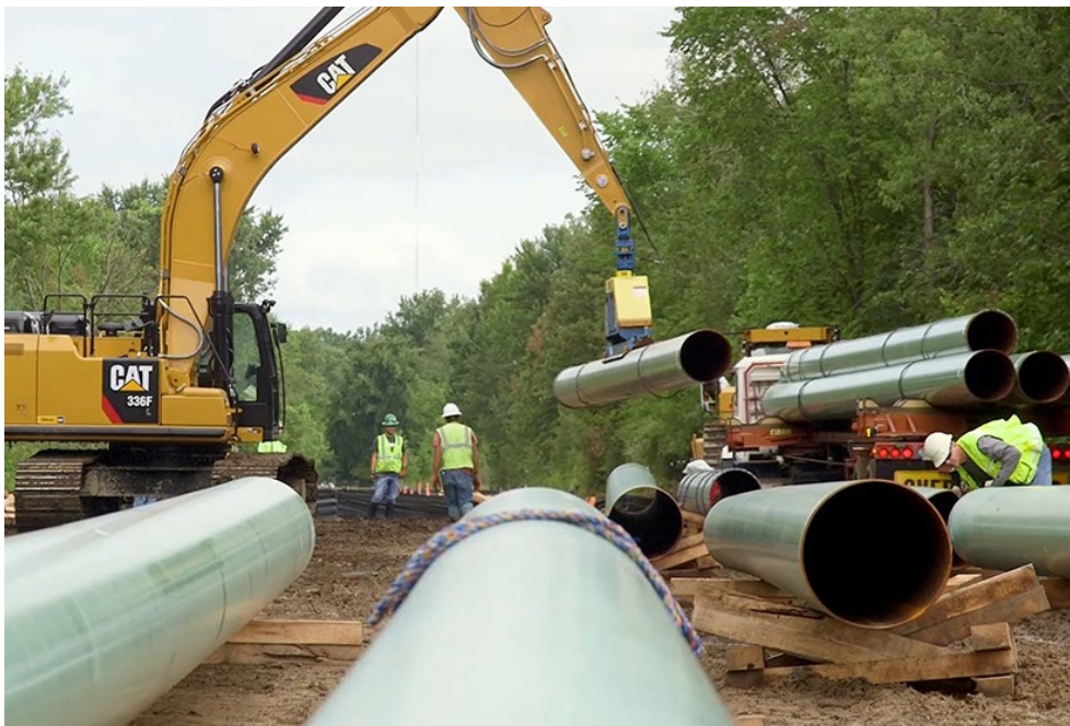
Construction of Consumer Energy’s Saginaw Trail pipeline project in Michigan | Consumers Energy
