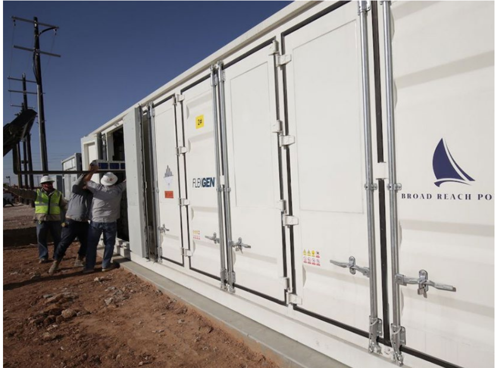
Broad Reach Power energy storage facility | Broad Reach Power
