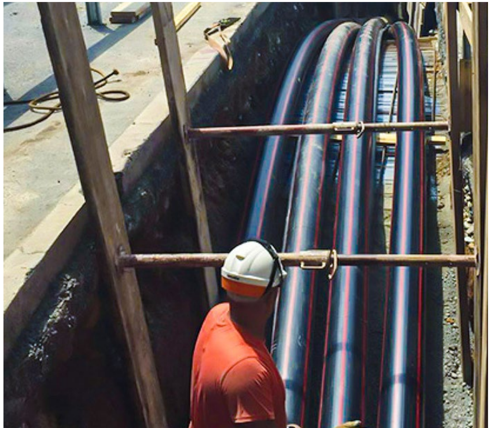
Buried HVDC cables in highway right of way (Italy-France Interconnector). | Roda S.p.A.
