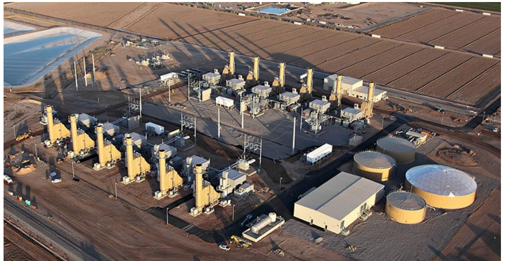
The 575 MW gas-fired Coolidge Generating Station is located on Arizona's Pinal County. | TC Energy
