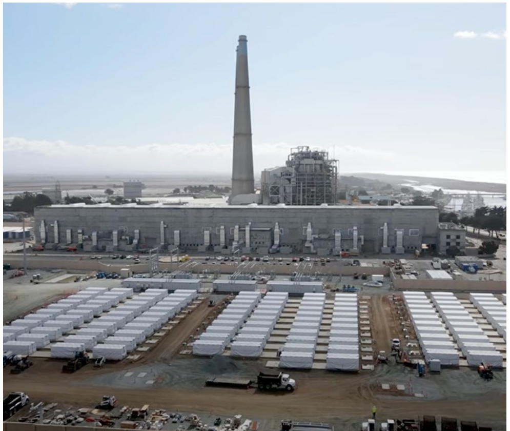
PG&E’s 182.5-MW Elkhorn Battery project was built next to Vistra’s 400-MW Moss Landing battery system on Monterey Bay in California. | EKM Metering
