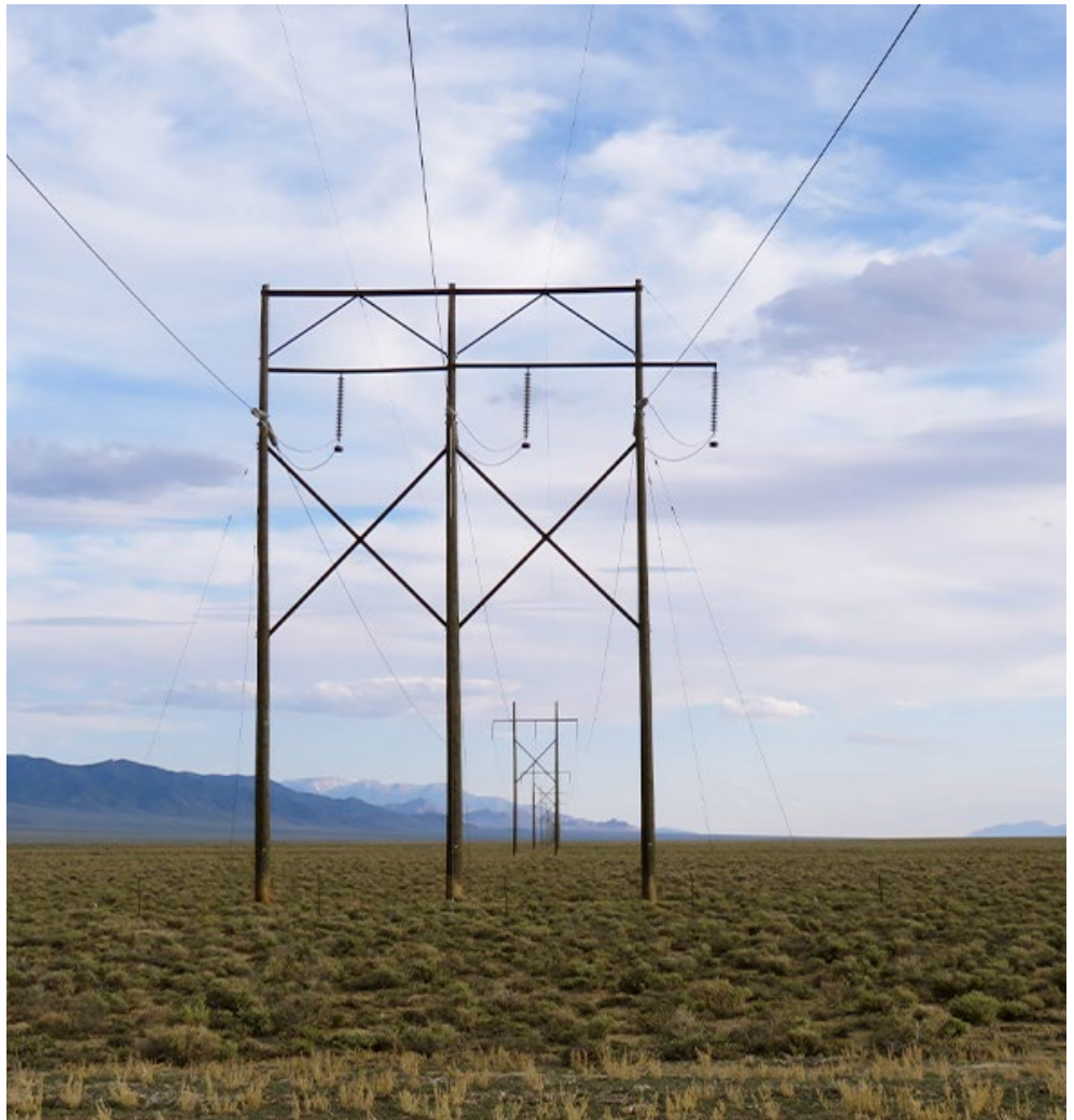
Transmission lines traverse a basin near Highway 50 in central Nevada. | © RTO Insider LLC
