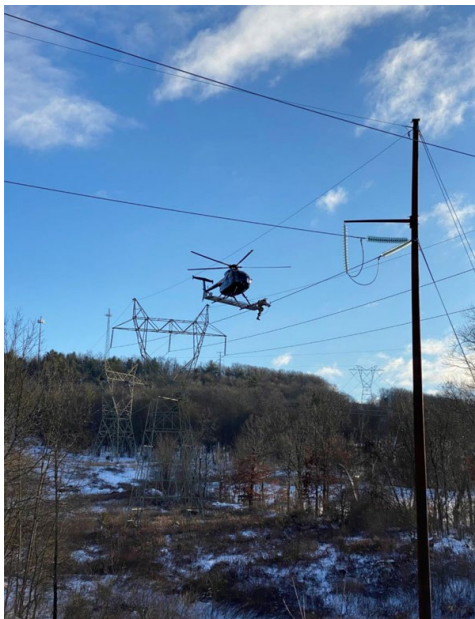
A PPL helicopter crew installs dynamic line rating sensors on transmission lines. | PPL
