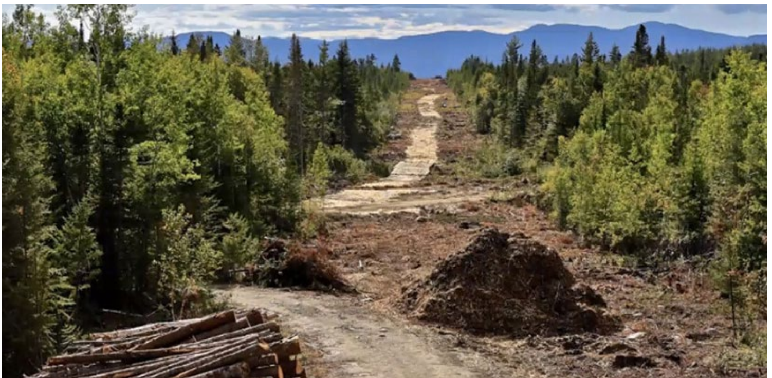
Gov. Janet Mills vetoed a transmission bill that its sponsor, Rep. Nicole Grohoski, says sprang from the public debate over the New England Clean Energy Connect project, seen under construction here. | Roger Merchant
