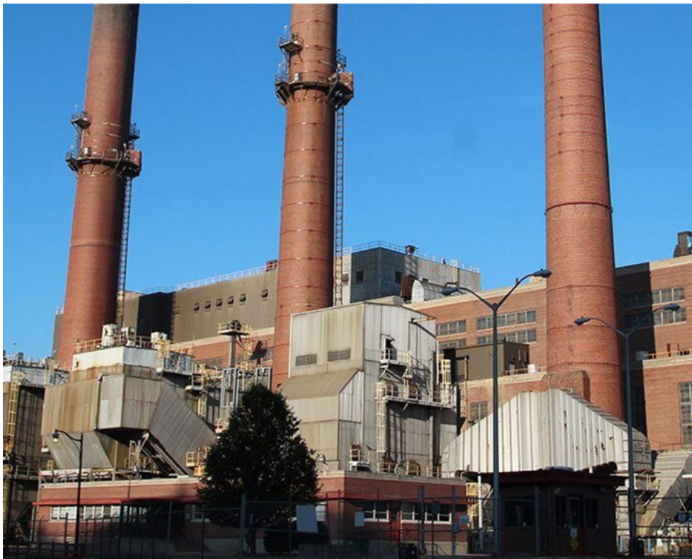
AES Indiana's Eagle Valley natural gas plant is offline because of disconnected wires and ruptured pipes at least until June. | AES Indiana
