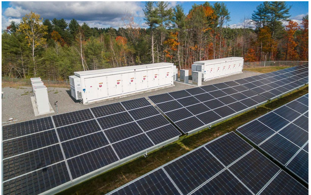
A Nexamp solar-plus-storage project in Massachusetts | Nexamp
