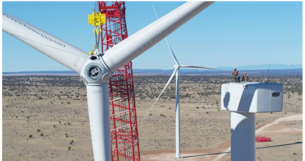
Pattern Energy completed construction in December on Western Spirit Wind, the largest renewable energy project in the U.S., with four wind farms totaling more than 1,050 MW in Guadalupe, Lincoln, and Torrance counties in central New Mexico. | Pattern Energy
