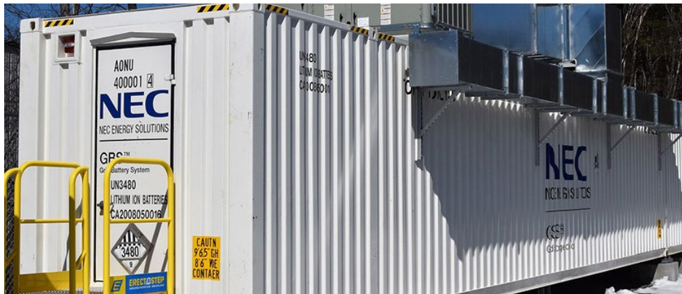
A storage project in Sterling, Mass. | Clean Energy Group
