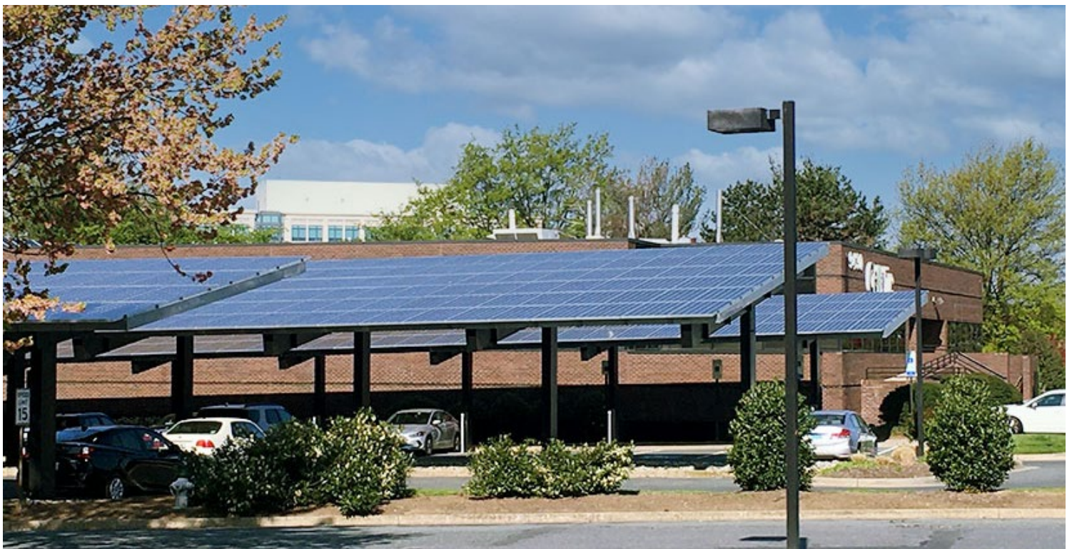
Solar panels over a parking lot in Rockville, Maryland | © RTO Insider LLC
