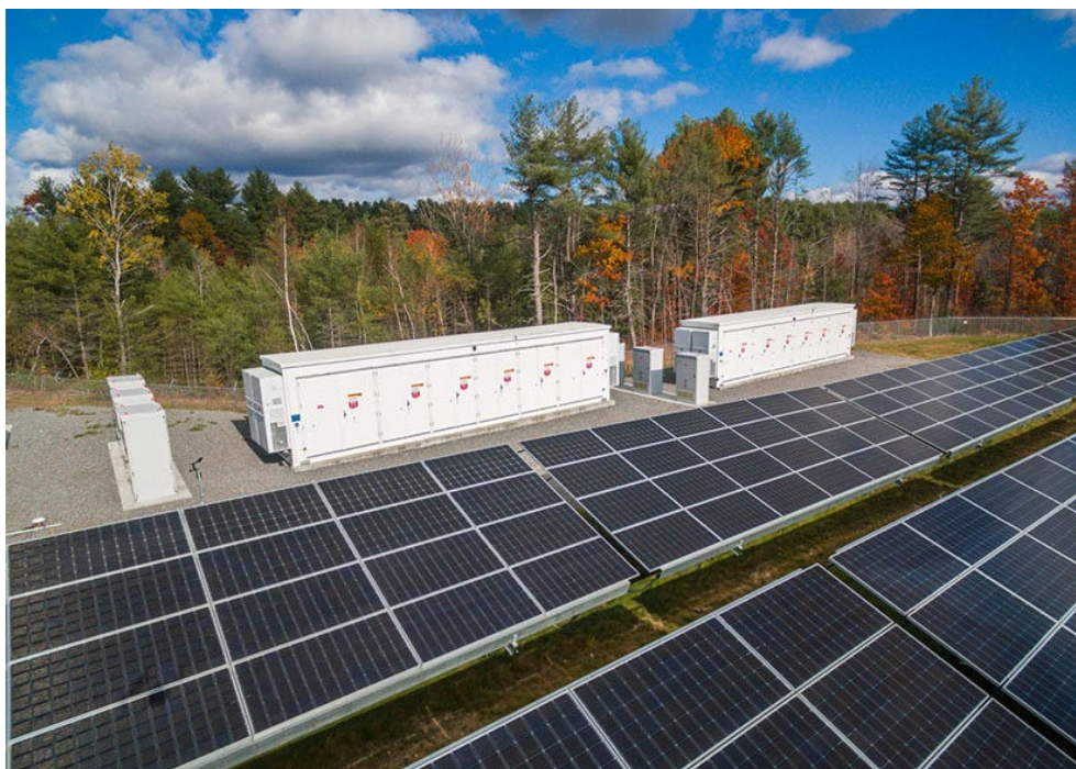
A Nexamp solar-plus-storage project in Massachusetts | Nexamp
