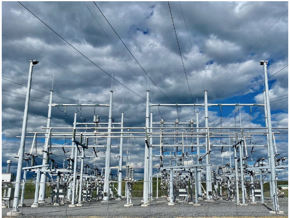
New York Transco rebuilt and, in June 2022, energized the Churchtown Switching Station in Claverack as part of a 22-mile transmission modernization project in the Hudson River Valley. | NY Transco
