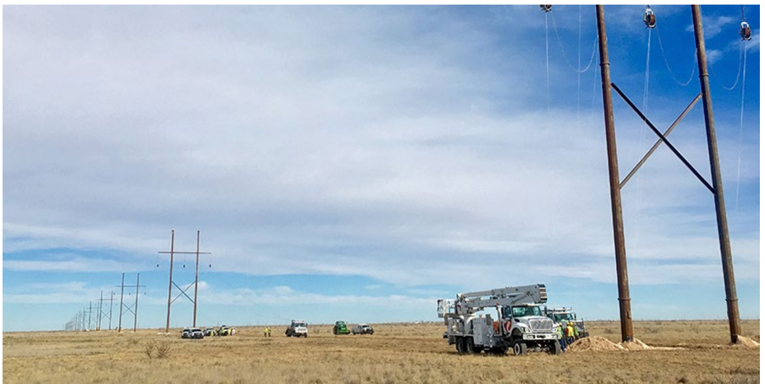
Xcel Energy service crews work on a new transmission line in West Texas. | Xcel Energy
