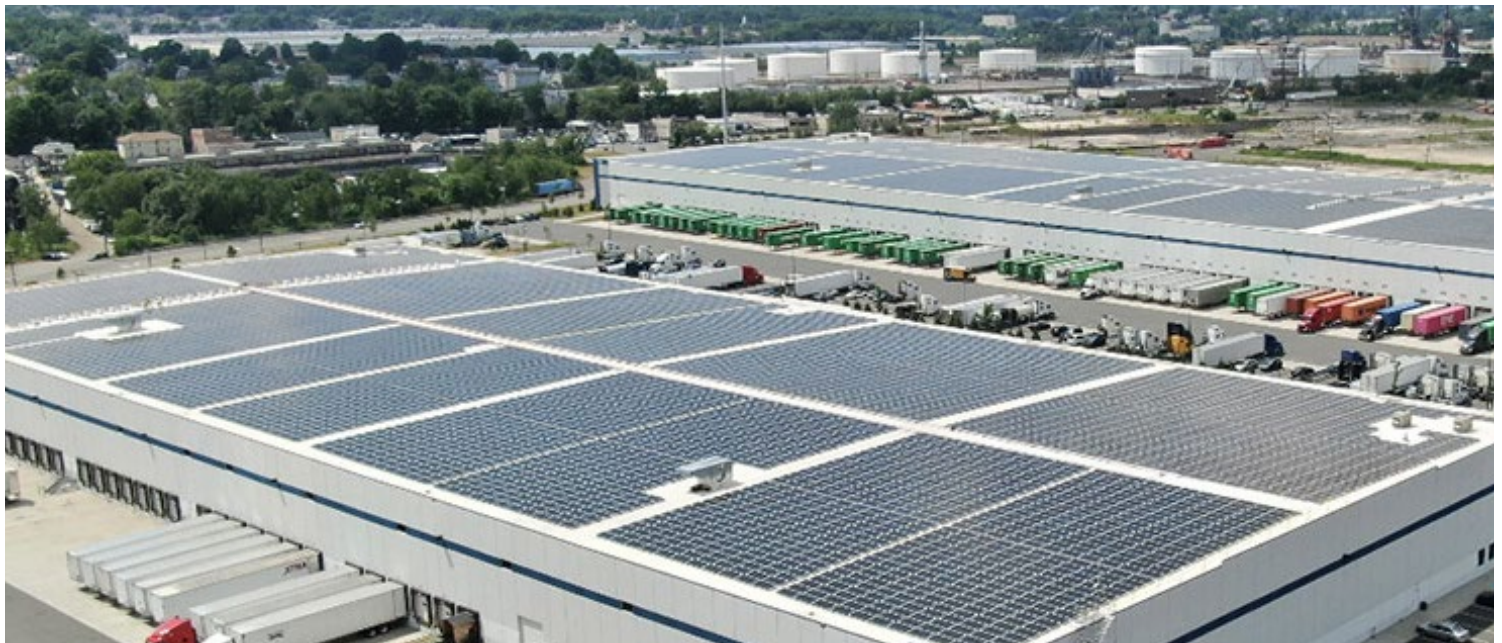
A solar project installed on a warehouse rooftop in Perth Amboy, N.J. | Solar Landscape
