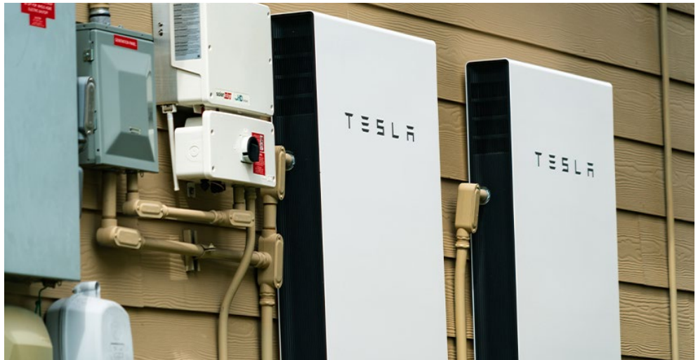
Up to 25,000 owners of Tesla Powerwall batteries could participate in PG&E’s pilot program. | Shutterstock
