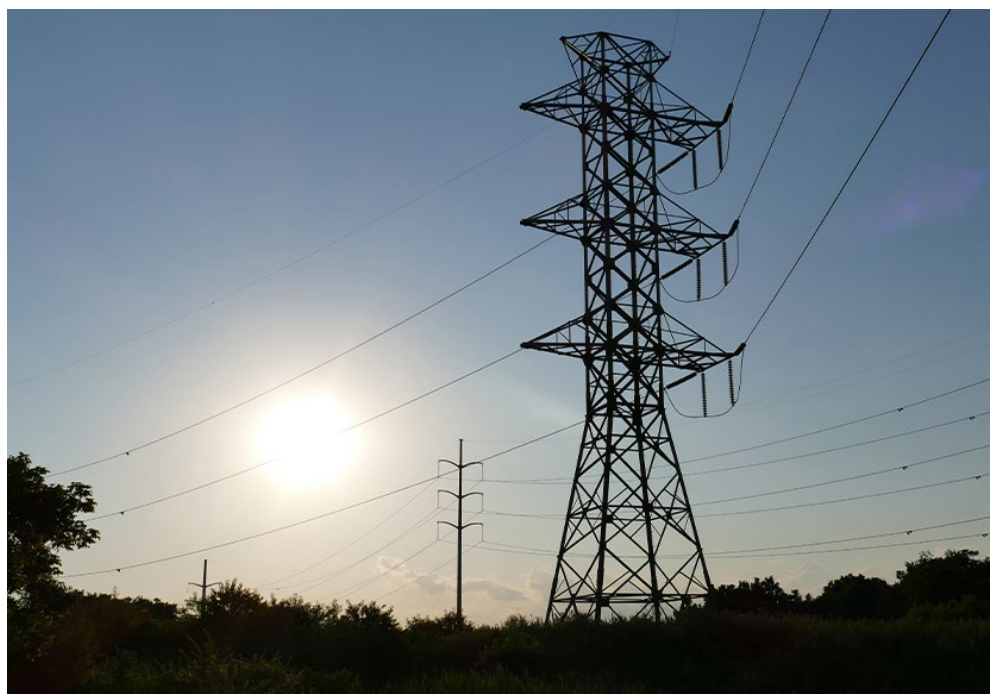
Transmission lines outside Wilmington, Del. | © RTO Insider LLC
