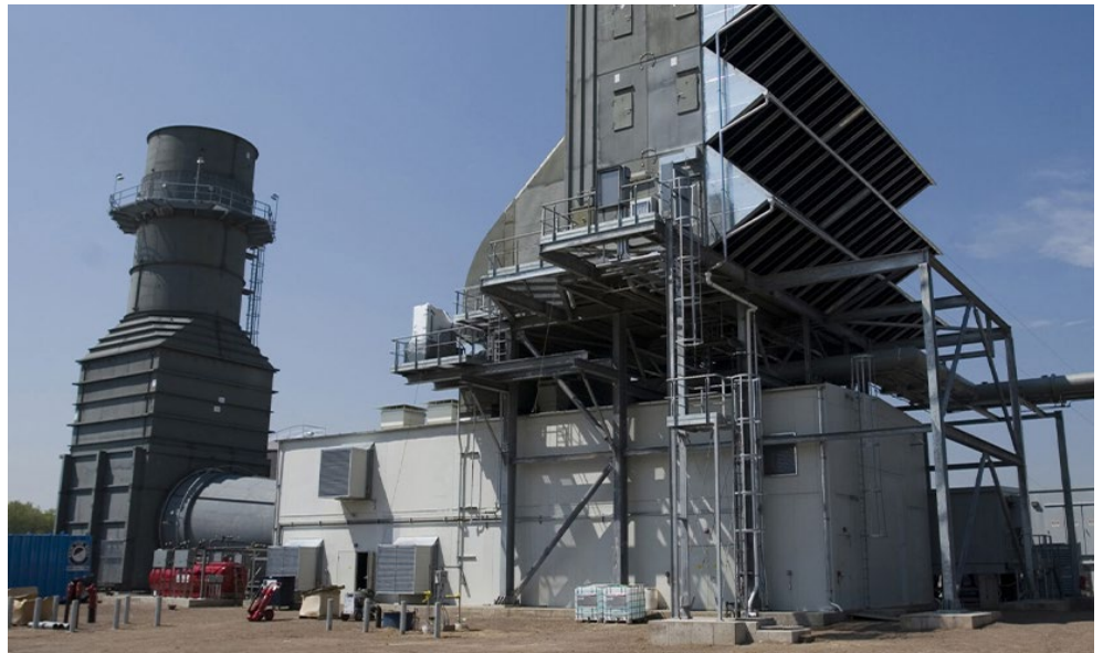
Great River Energy's natural gas-fired Cambridge Station in Minnesota | GRE
