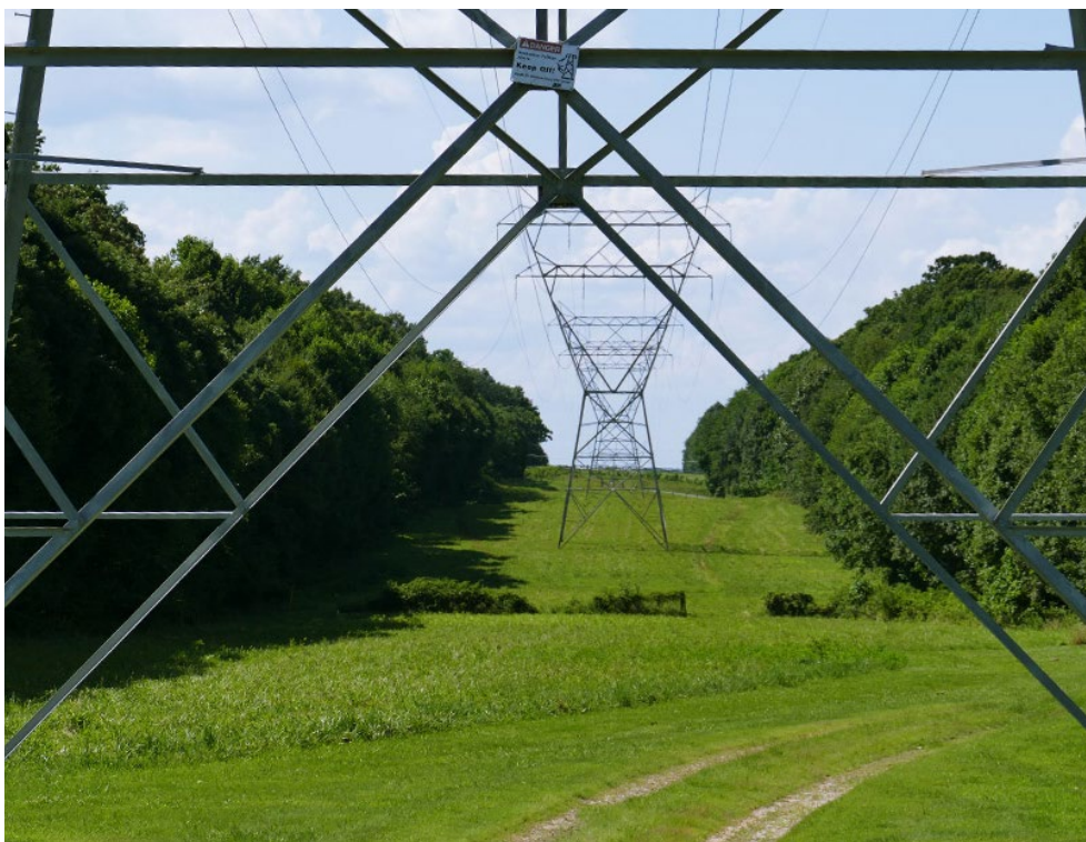
PJM transmission line near Conowingo Dam | © RTO Insider LLC
