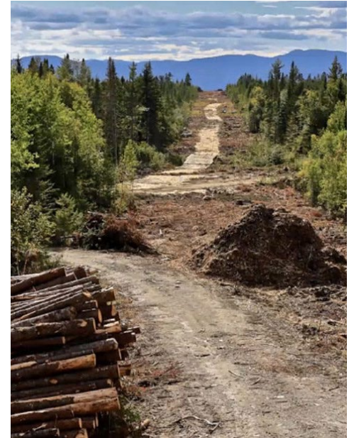
A group of individuals and entities lost their appeals of Central Maine Power's permit for the NECEC transmission line, seen under construction here. | Roger Merchant
