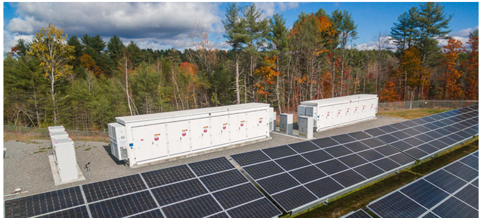
A Nexamp solar-plus-storage project in Massachusetts | Nexamp
