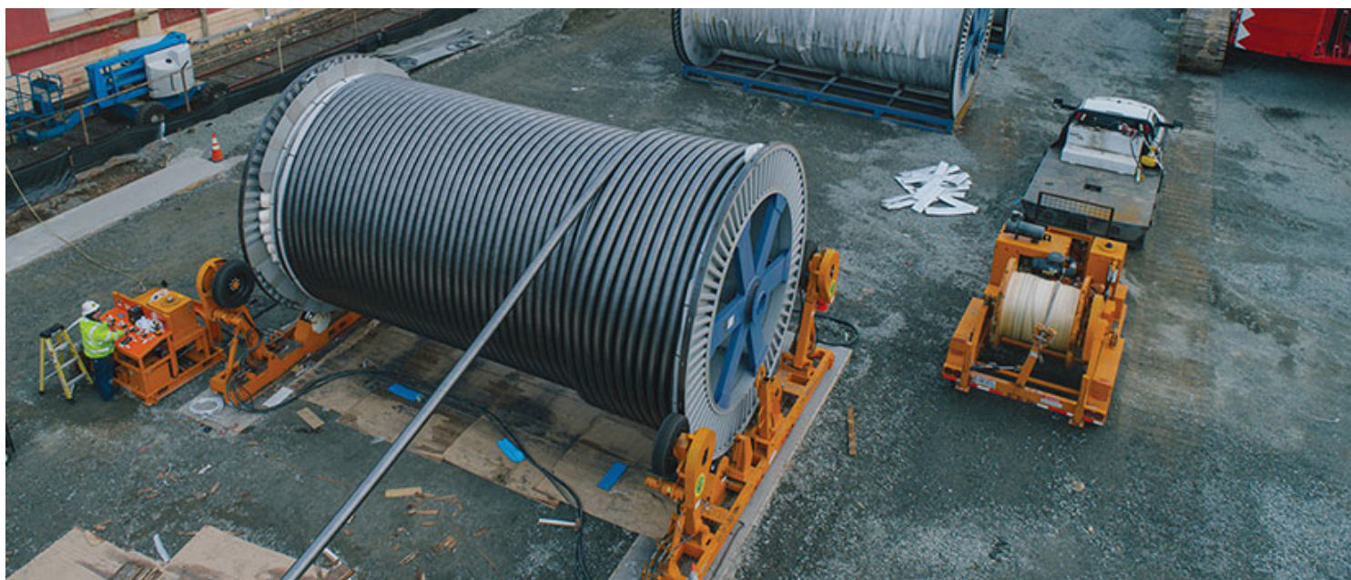
Power Engineers said its work on the underground transmission project in the Bergen-Linden Corridor required a 6,600-foot-long trenchless crossing of Newark Bay, the longest horizontal directional drilling project for 345-kV cable in North America. | Power Engineers
