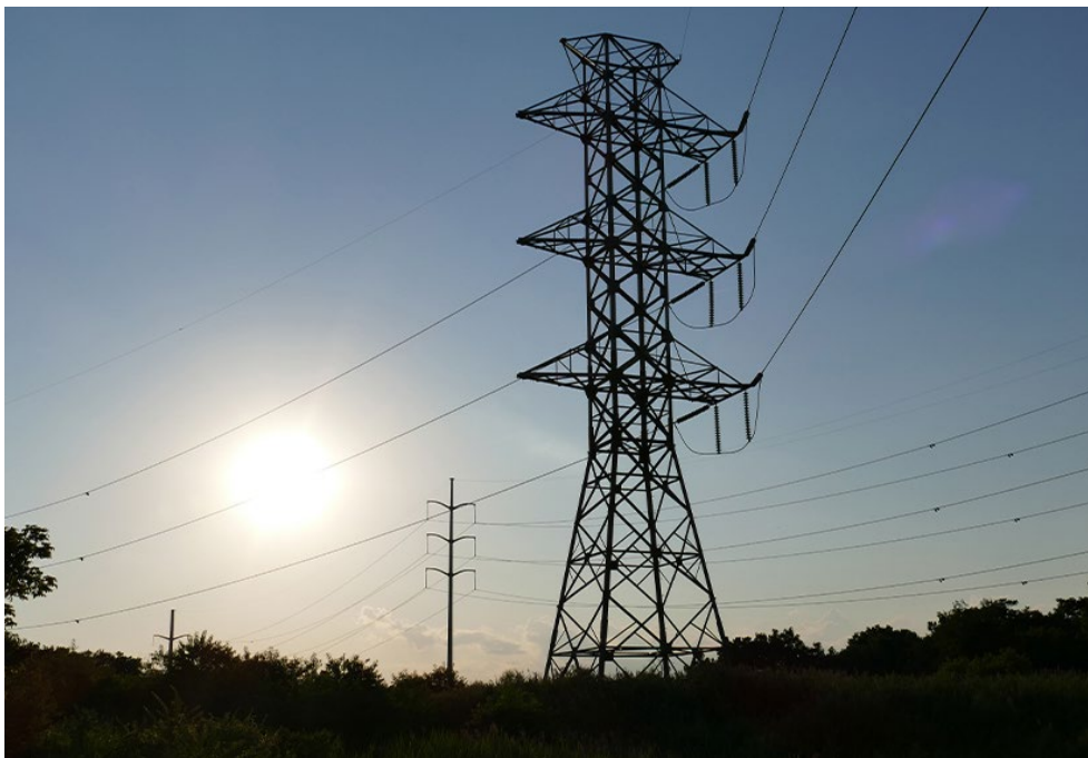
Transmission lines in Wilmington, Del. | © RTO Insider LLC
