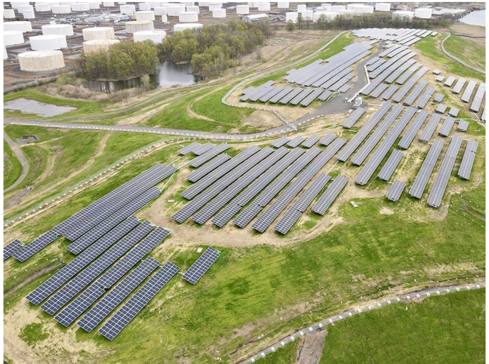
Navisun's 4.5-MW Linden Hawk Rise community solar project, located on a former landfill site in Linden, N.J. | Navisun
