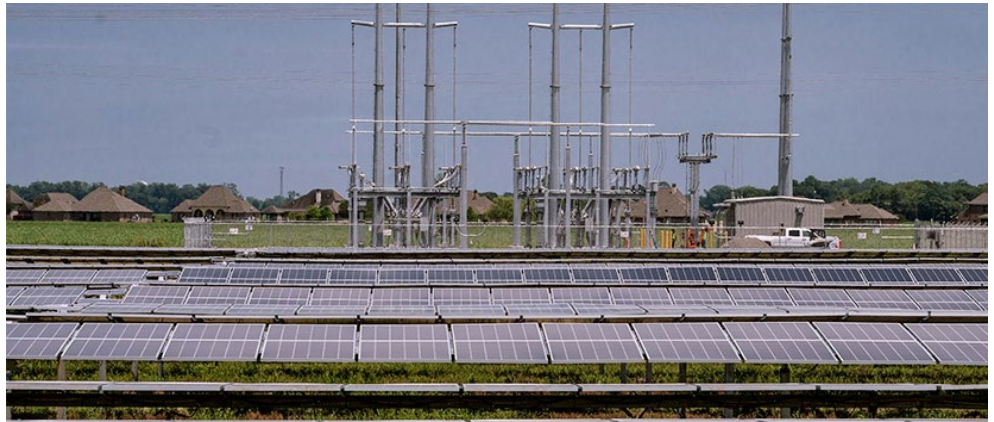
Solar farm in West Baton Rouge Parish | Entergy
