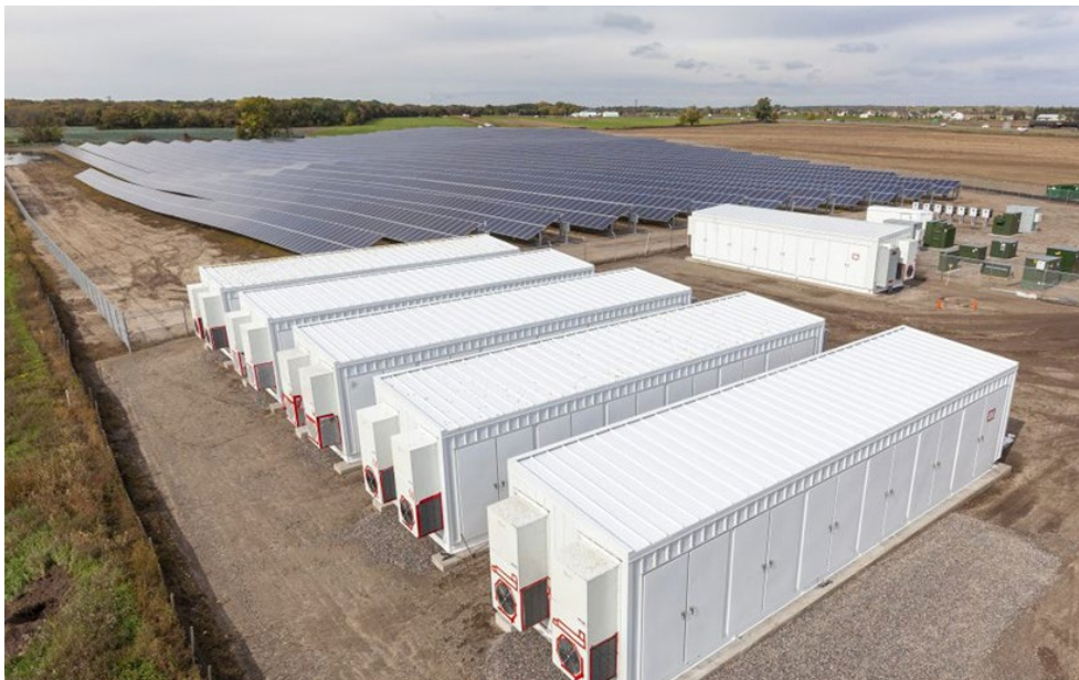
Connexus Energy solar and storage site in Minnesota | Connexus Energy
