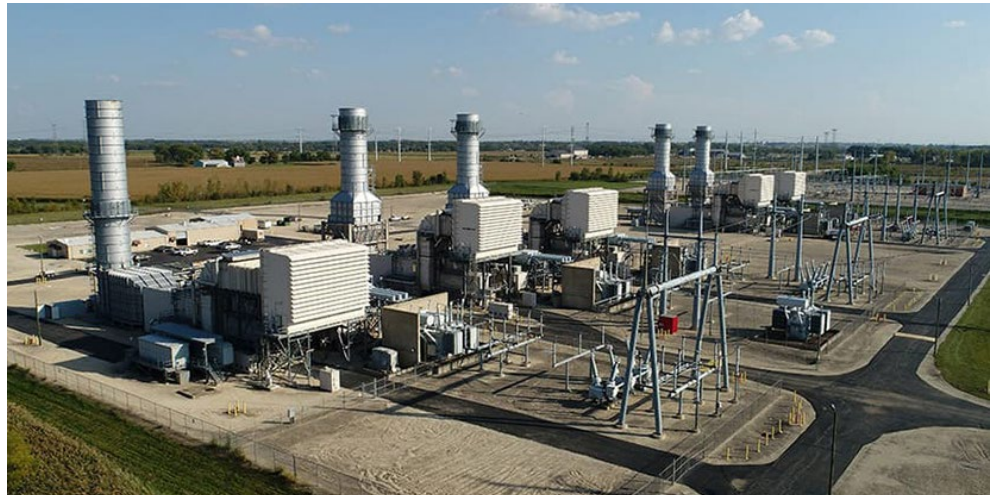
Elwood Power Plant | J-Power USA
