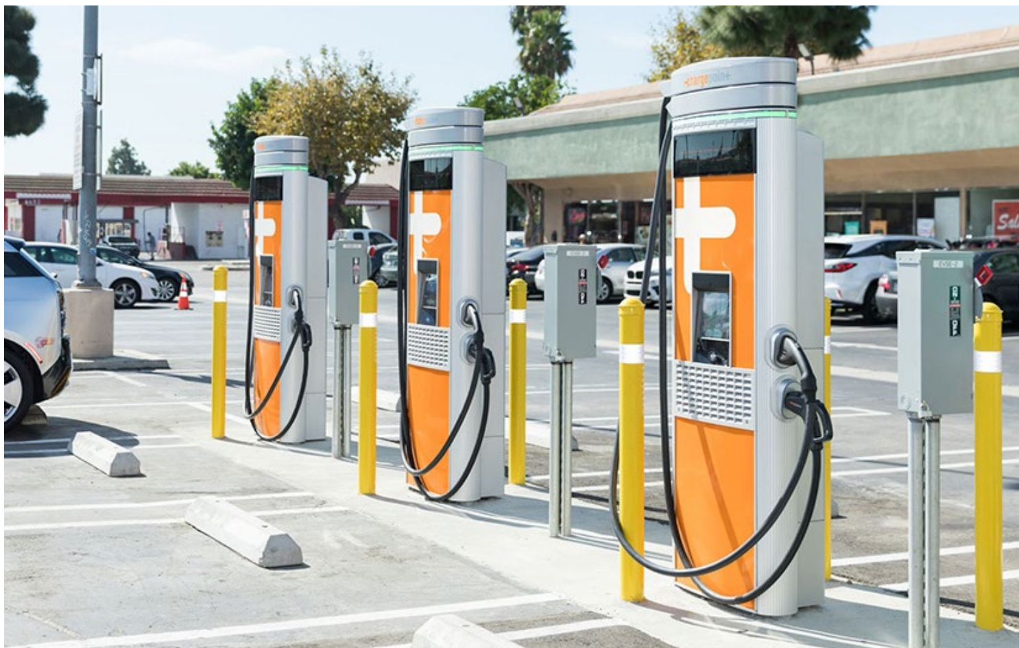
ChargePoint CPE250 fast charger at a plaza in Southern California | ChargePoint
