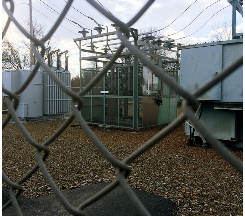
PECO substation near PJM headquarters | © RTO Insider LLC
