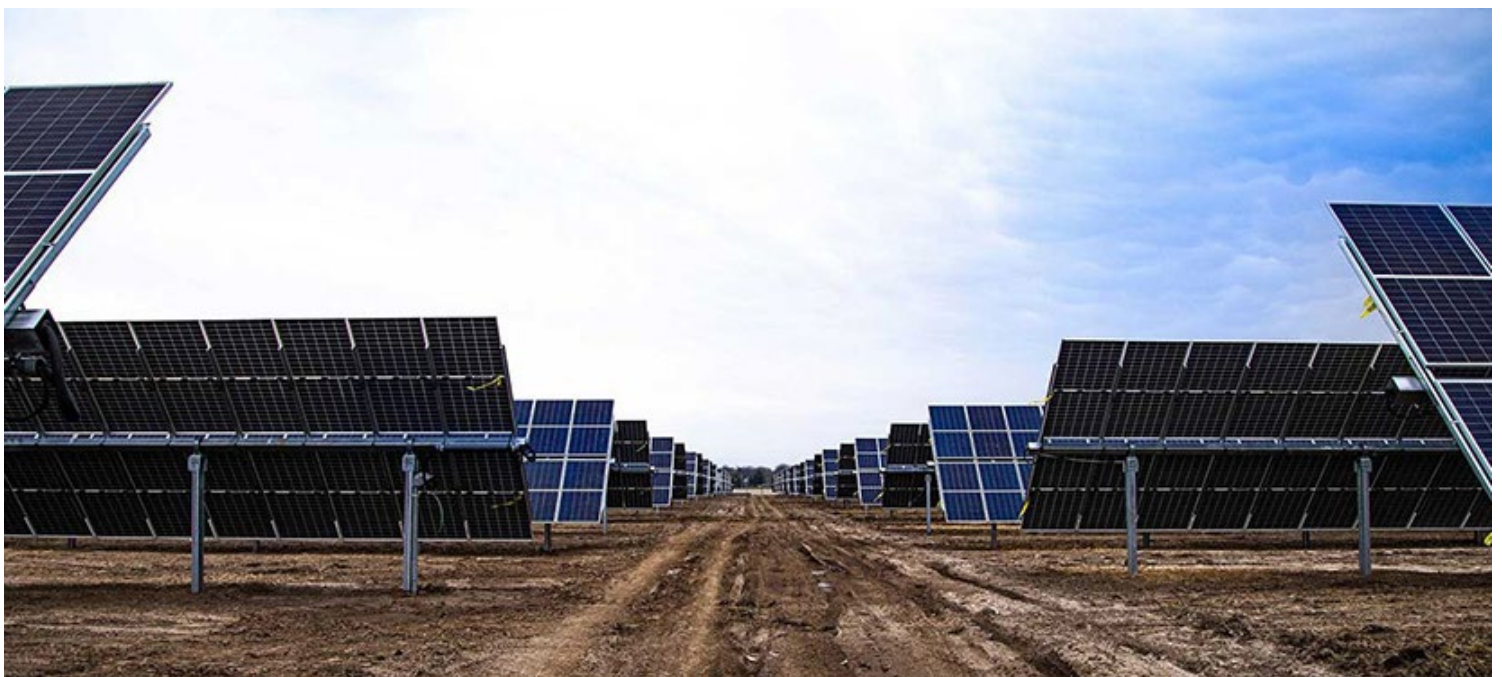
The O'Brien Solar Fields in Fitchburg, Wisc. | Madison Gas and Electric
