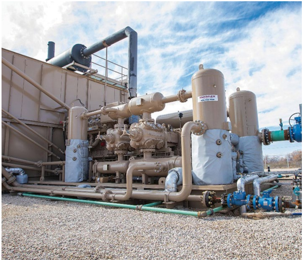
Natural gas compressor | Ariel Corp.
