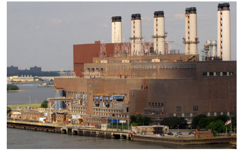
Astoria Generating Station in Queens | Ben Schumin, CC BY-SA-2.0, via Wikimedia
