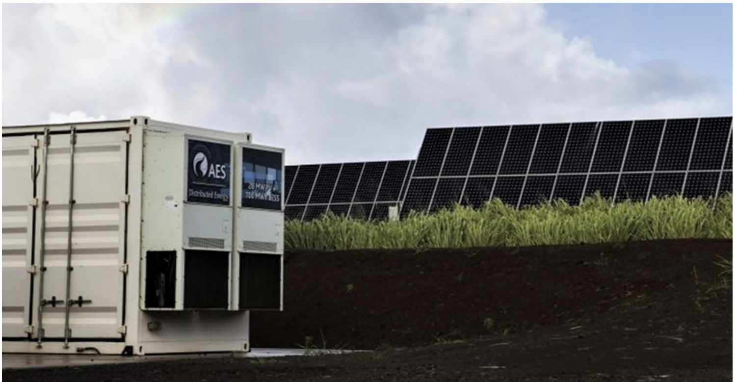
AES Lawai solar and storage project | National Renewable Energy Laboratory
