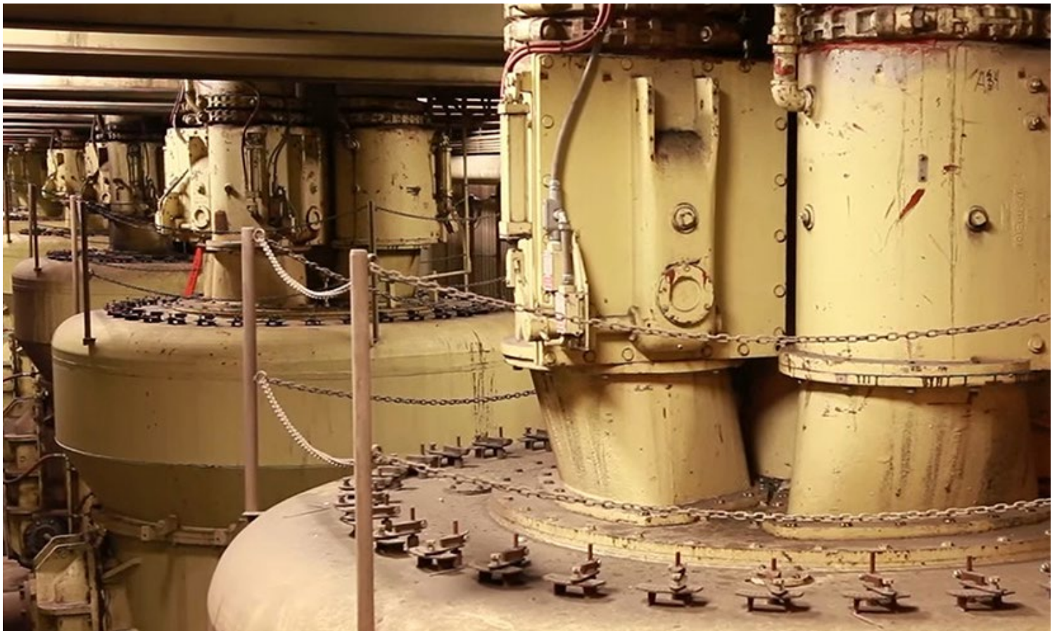
Interior of the Tolk Generating Station | Xcel Energy
