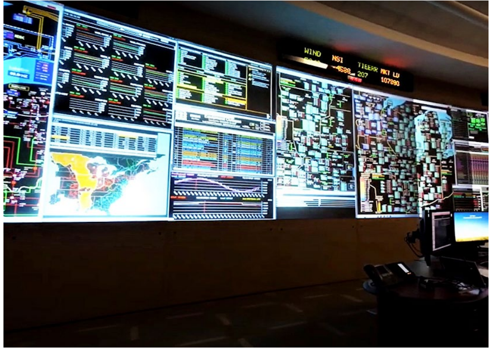
MISO control room | MISO
