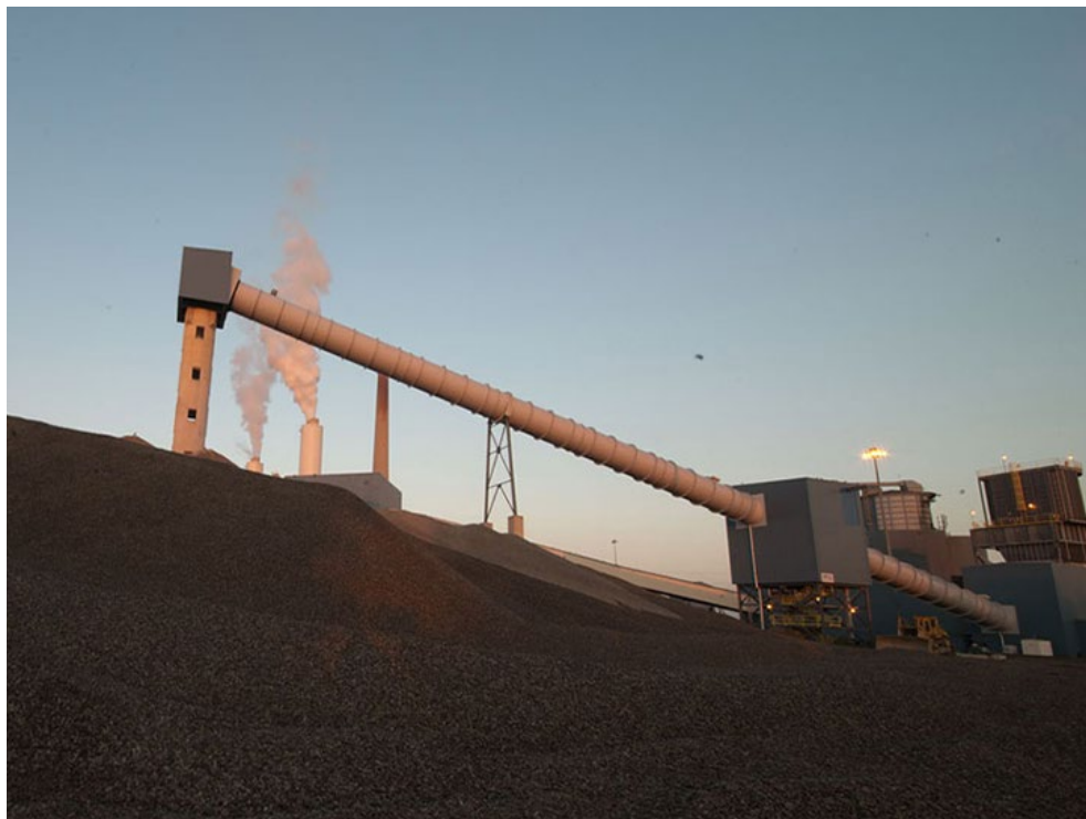
The Monroe Power Plant, one of the largest coal-fired generators in the U.S., will close by 2028. | DTE Energy
