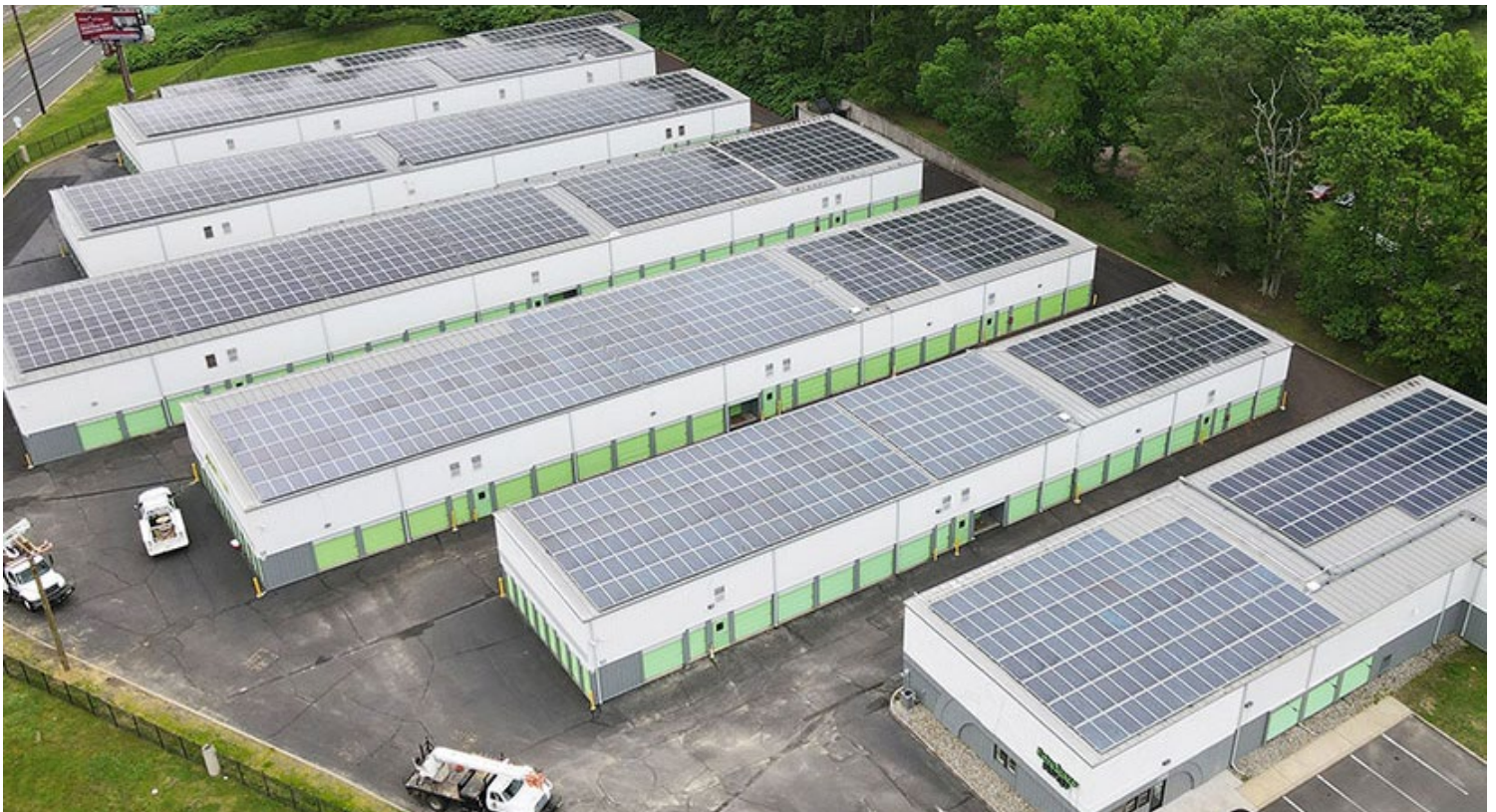
A 500-kW community solar project covering commercial rooftops in Neptune Township, N.J., will provide enough clean electricity to power 1,400 homes. | Solar Landscape
