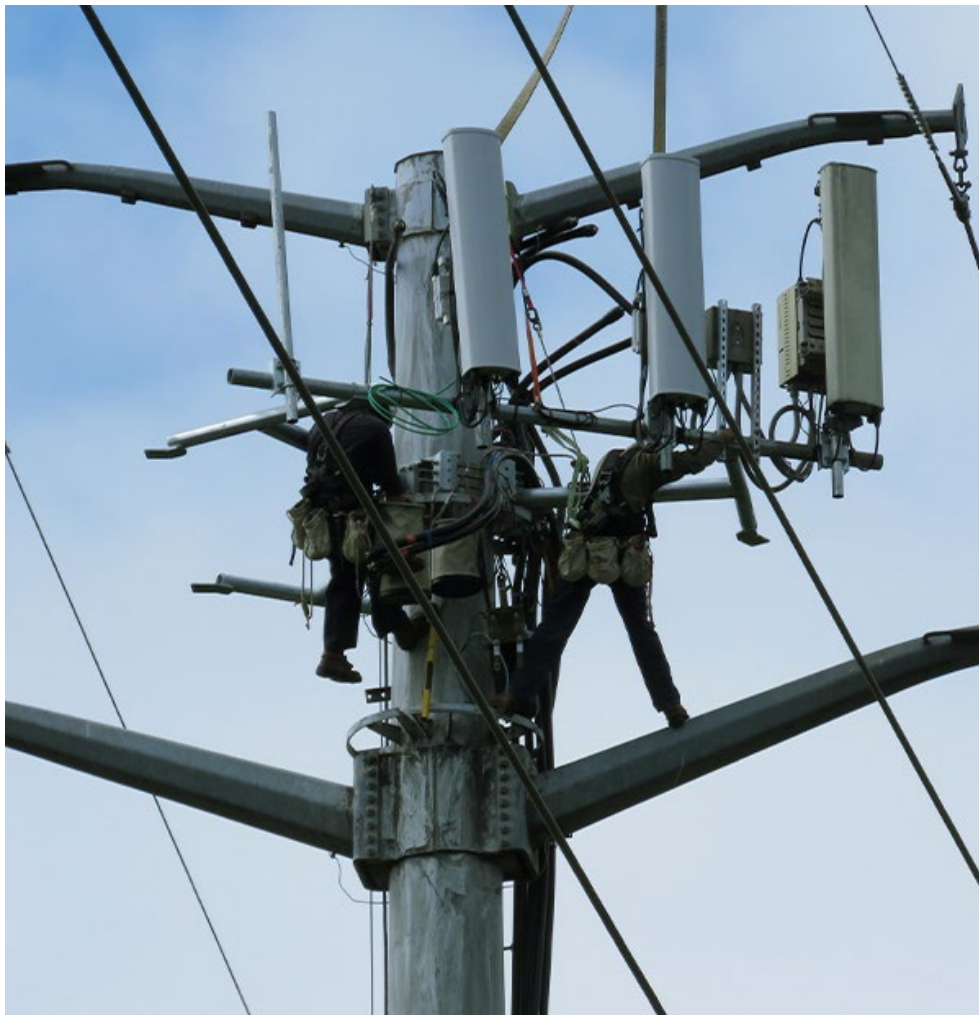
Repair work on a PEPCO transmission line in Potomac, Md. | © RTO Insider LLC
