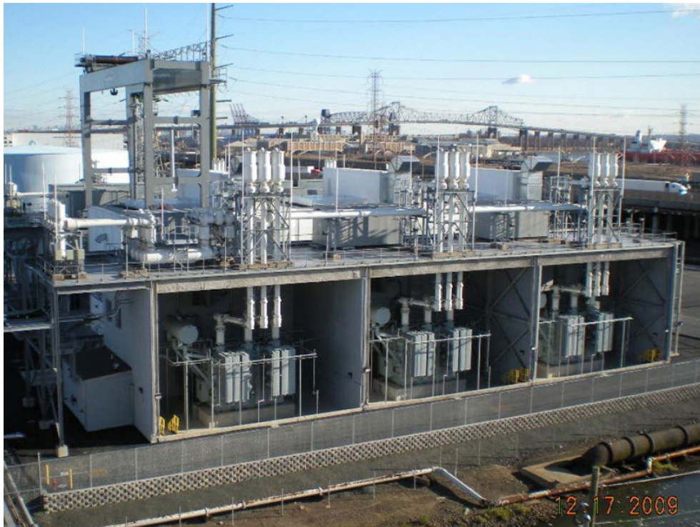
Linden VFT delivers power from its only customer, PSEG Energy Resources & Trade, to its facilities near the PJM border. | DCO Energy
