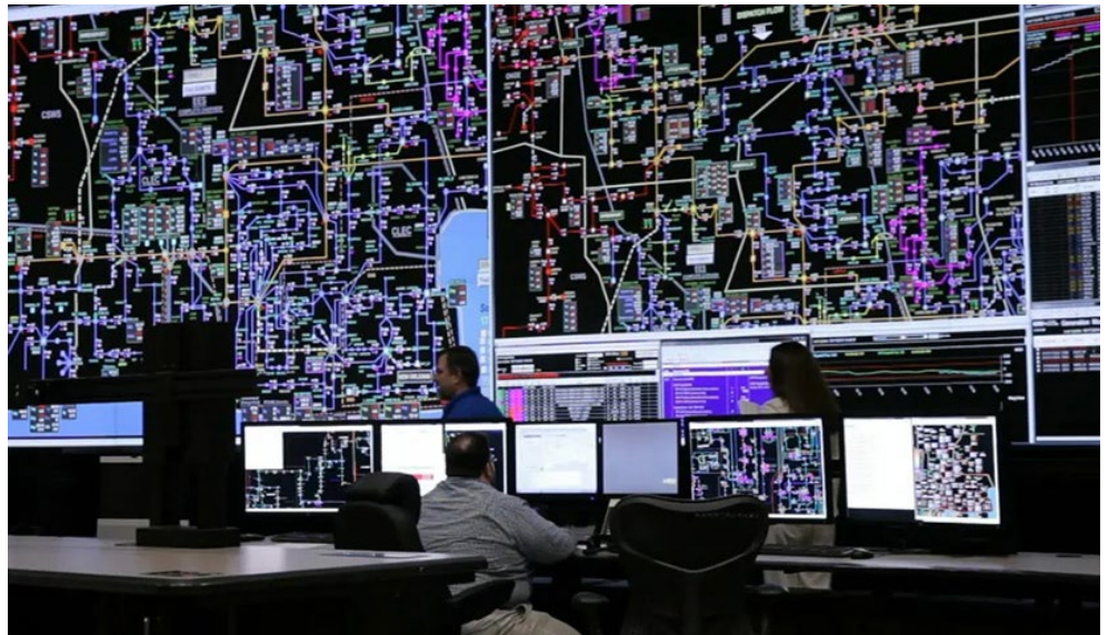
MISO control room | MISO
