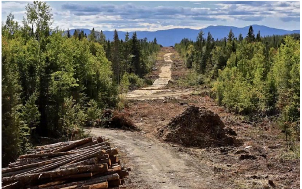
A portion of the right of way for the New England Clean Energy Connect transmission line | Roger Merchant
