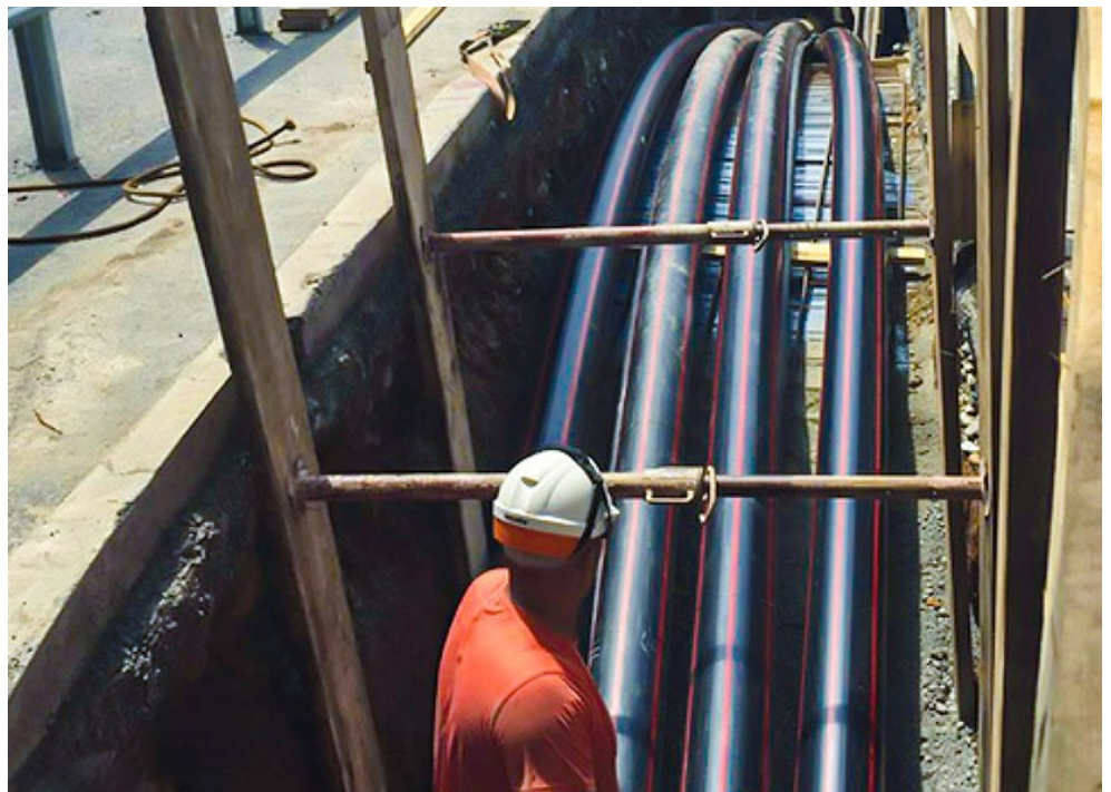
Buried HVDC cables in a highway right of way (Italy-France Interconnector) | Roda S.p.A.
