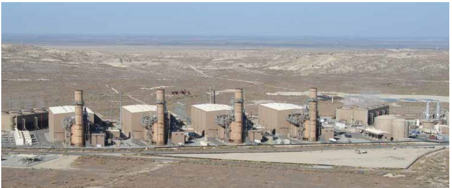
La Paloma Generating Plant in Kern County, Calif. | MeeFog
