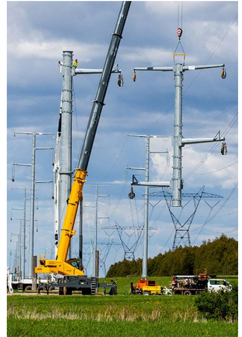
NYPA works on the Moses-Adirondack Smart Path Reliability Project. | New York Power Authority
