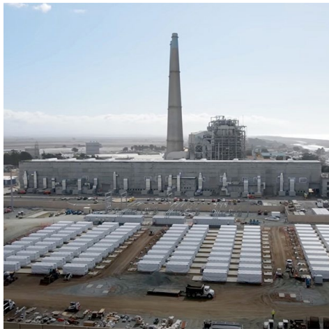
The assets PG&E plans to sell include the 182.5-MW Elkhorn Battery project, one of the world’s largest battery arrays, on California’s Monterey Bay. | EKM Metering
