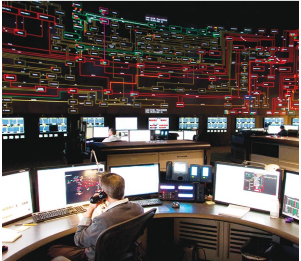
NYISO control room in Rensselaer, N.Y. | NYISO
