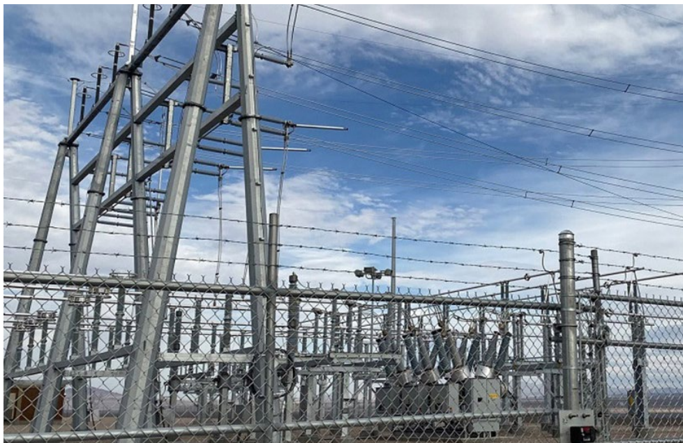
FERC has rejected a GridLiance rehearing request over the classification of distribution facilities in Oklahoma's Panhandle. | GridLiance
