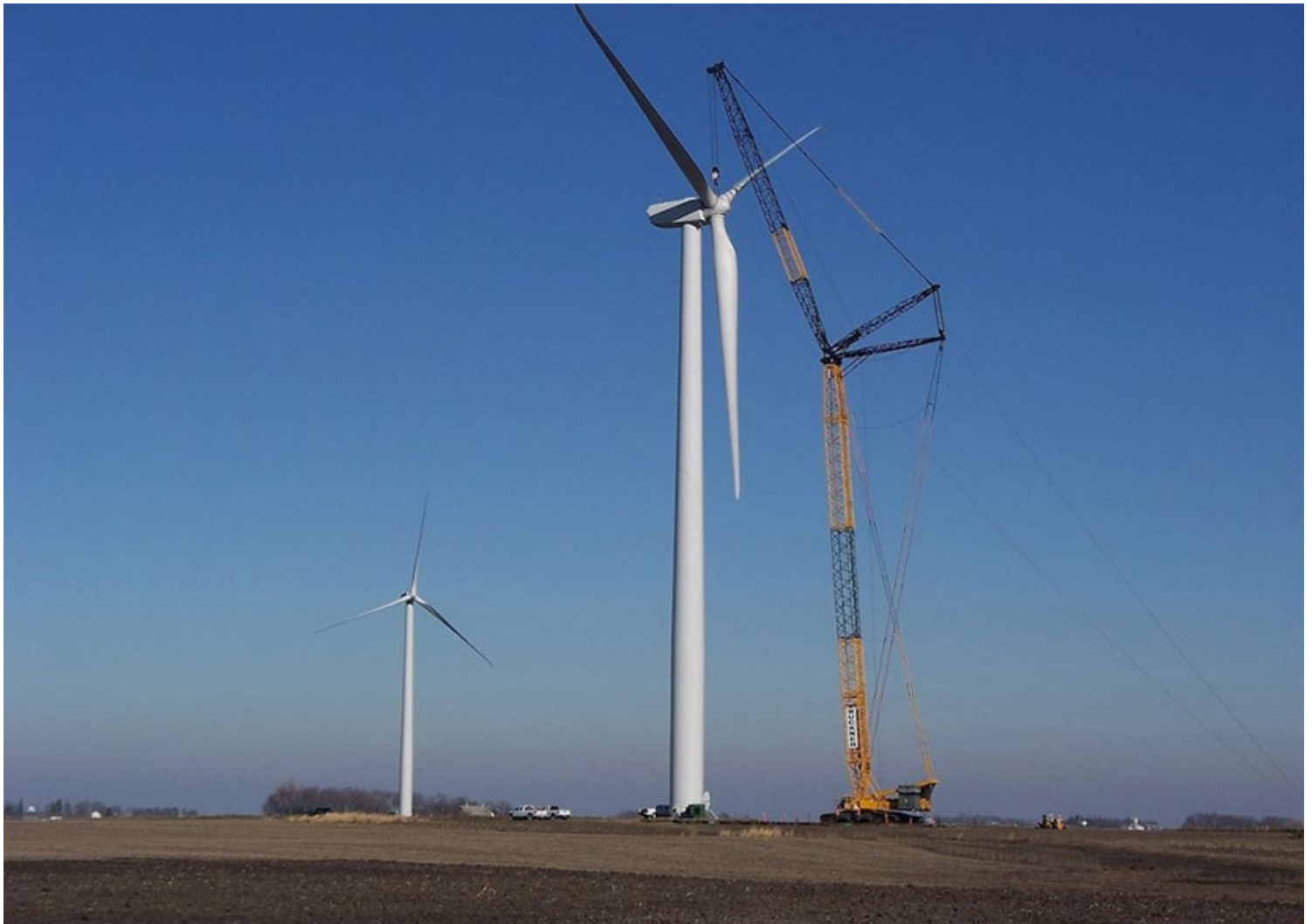
The 198 MW Pomeroy Wind Project in Iowa | EDF Renewables
