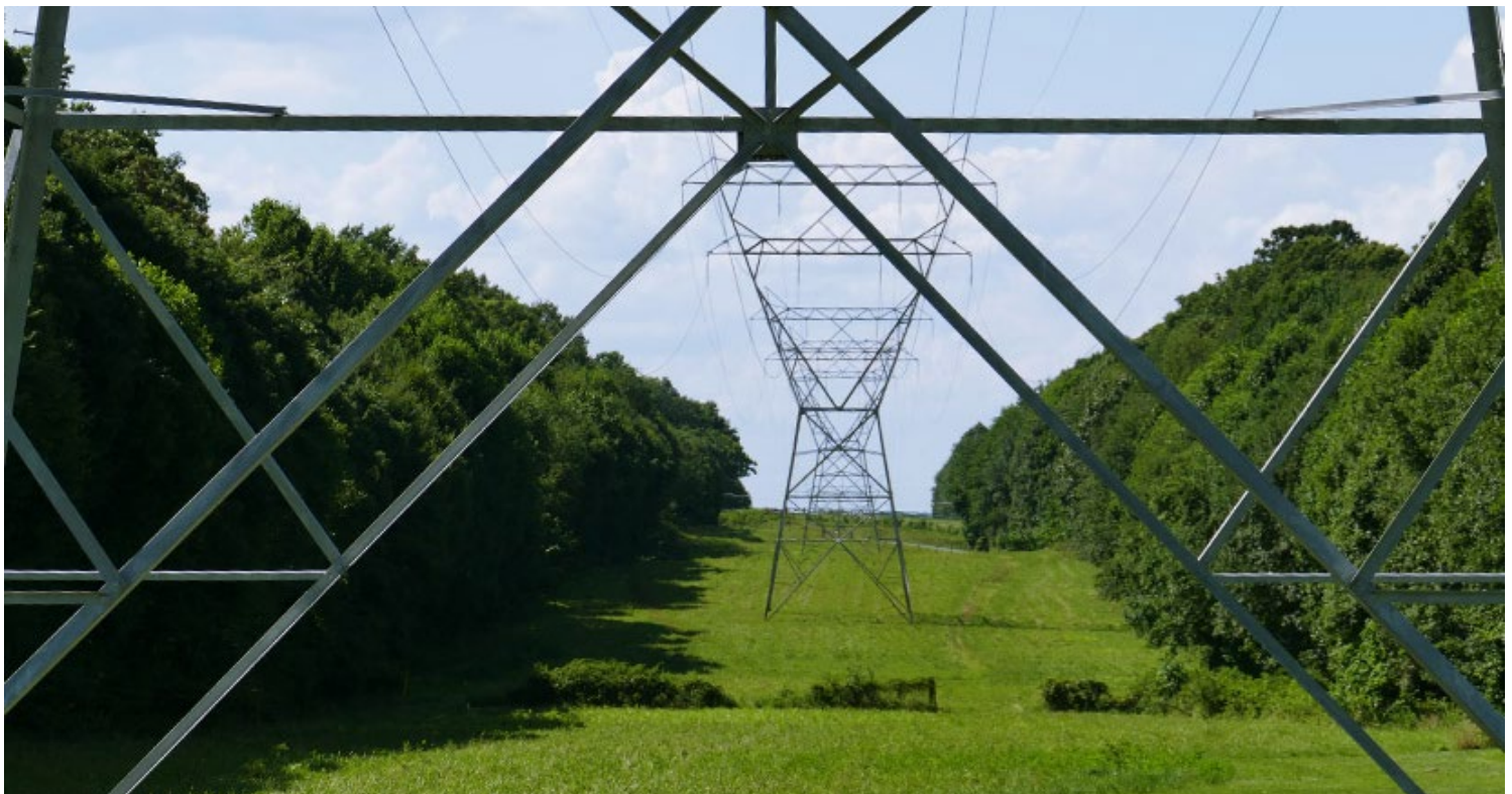
PJM transmission line near Conowingo Dam | © RTO Insider LLC
