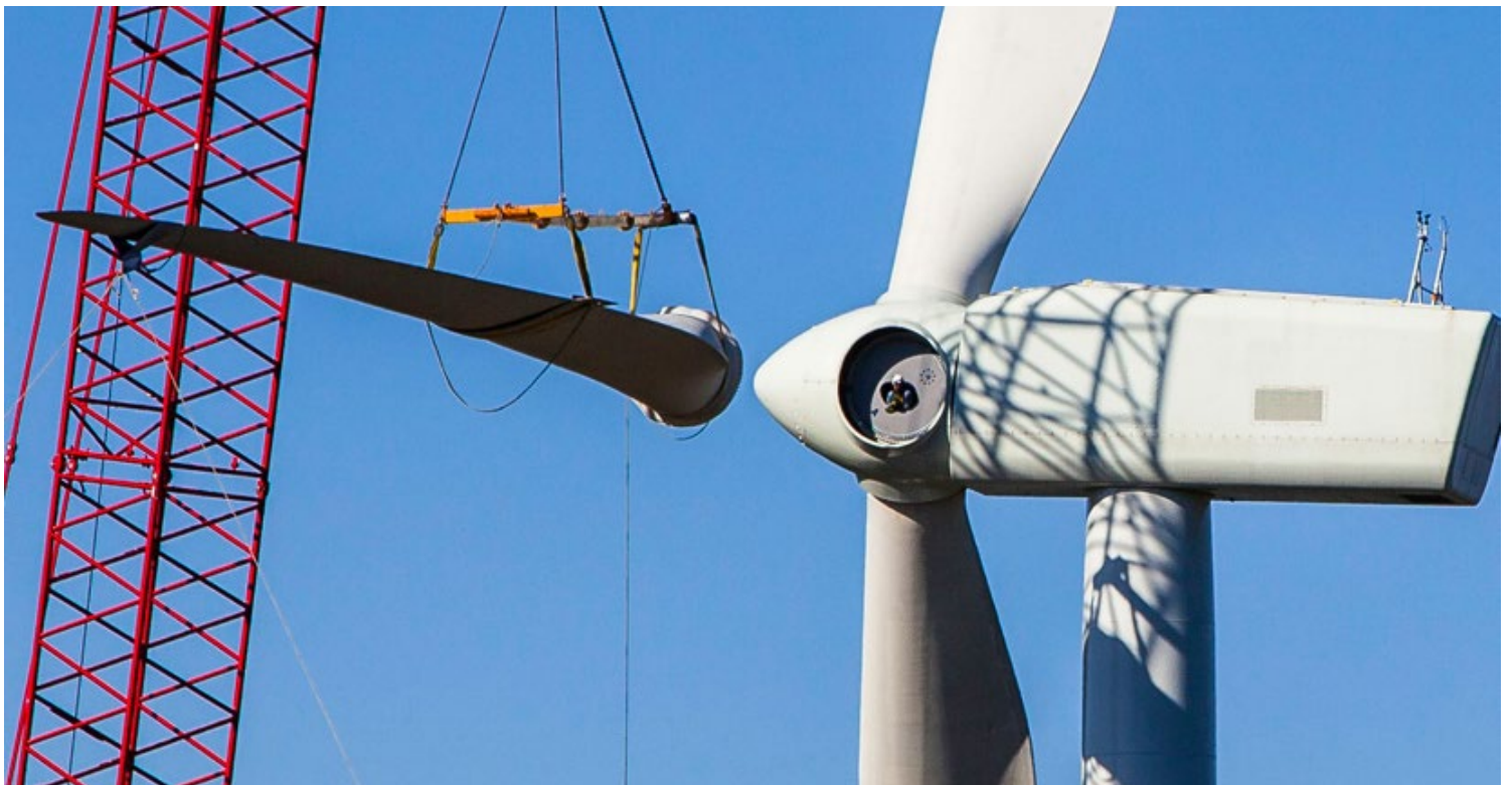
A wind turbine is assembled at an Avangrid project in Groton, N.H. | Avangrid
