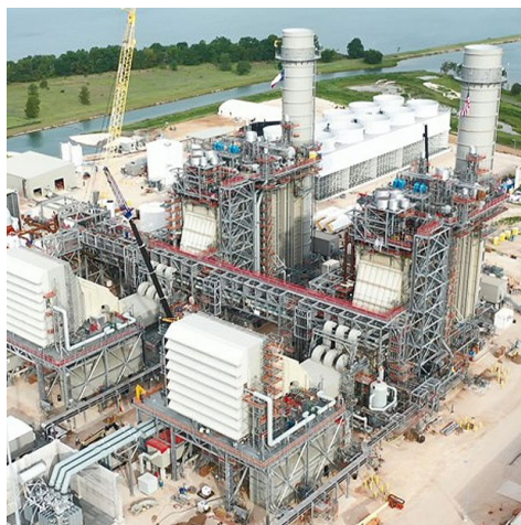
Entergy Texas' Montgomery County Power Station was cited as one of the reasons the Hartburg-Sabine line is no longer necessary. | Entergy
