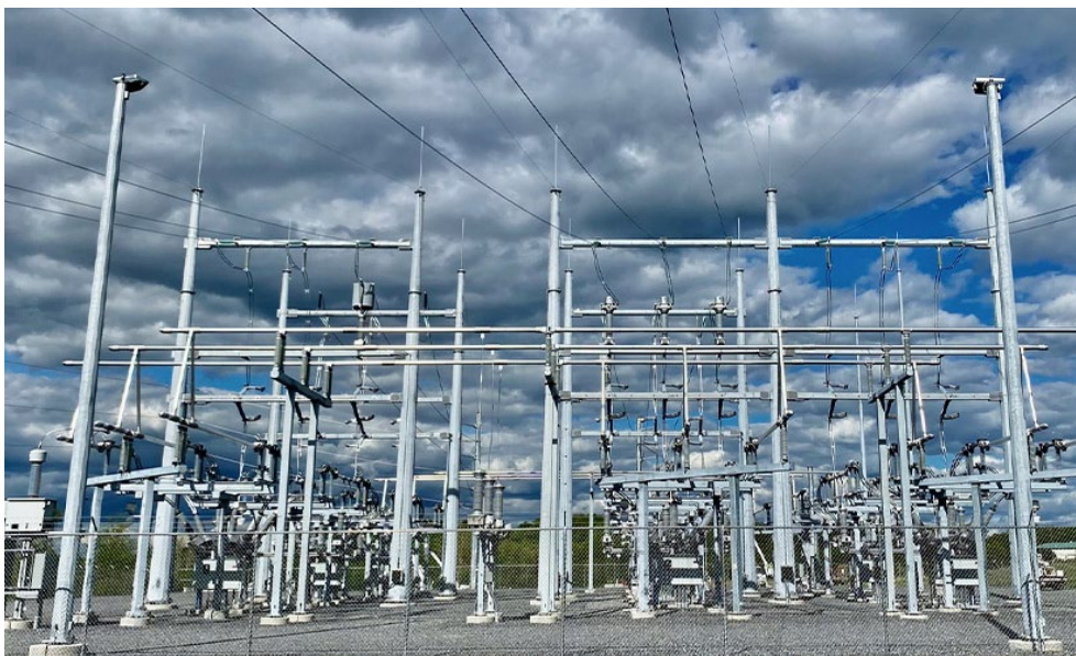
New York Transco rebuilt and in June 2022 energized the Churchtown Switching Station in Claverack as part of a 22-mile transmission modernization project in the Hudson River Valley. | NY Transco
