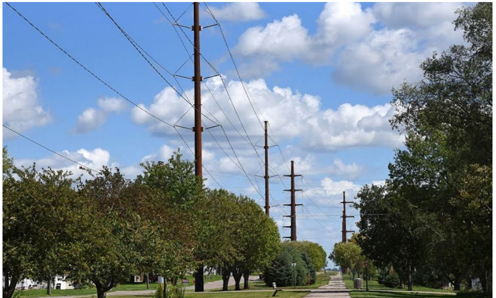
ITC Midwest's Traer-Dysart 161-kV line in Iowa | ITC Holdings
