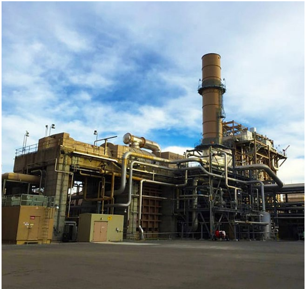
NV Energy's new gas-fired peaker facility will be built at the site of the Silverhawk Generating Station in Southern Nevada. | Lochsa Engineering
