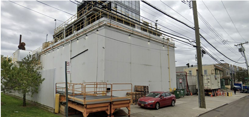
Cubit Power One's 11 MW combined heat and power generation facility in Staten Island | Google
