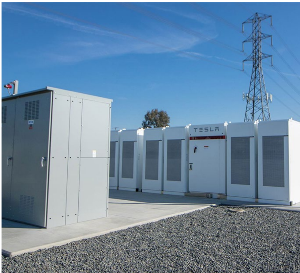
Batteries need to be available during summer shortfalls, CAISO said. | Southern California Edison
