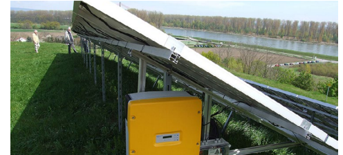
Inverter-based resource with electronic power converter | Claus Ableiter, CC BY-SA 3.0, via Wikimedia Commons
