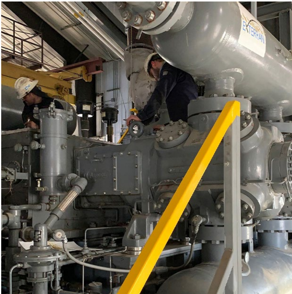
Interior of a NorthWestern Energy gas plant in Montana | NorthWestern Energy
