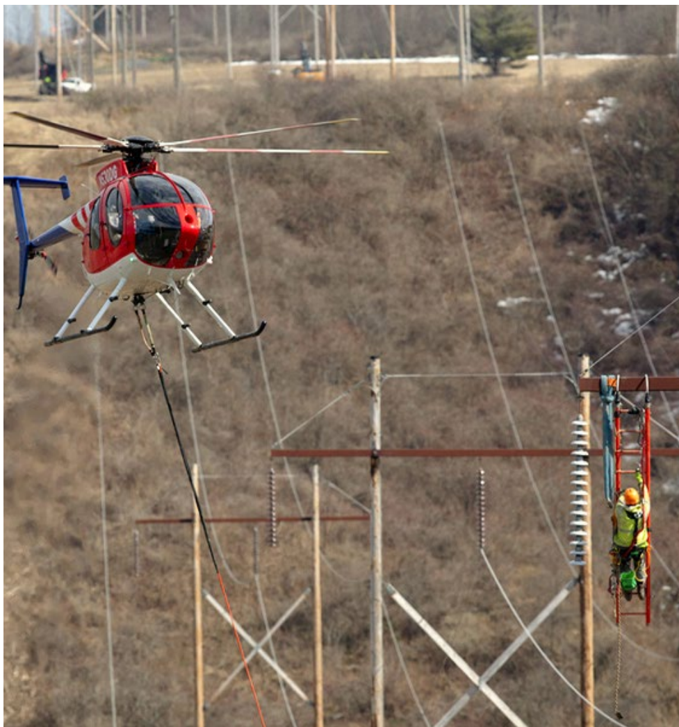
Work continues on the Central East Energy Connection upgrade near Schenectady, N.Y., in late March. | NYPA
