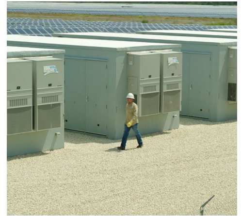
NextEra Energy battery storage | NextEra
