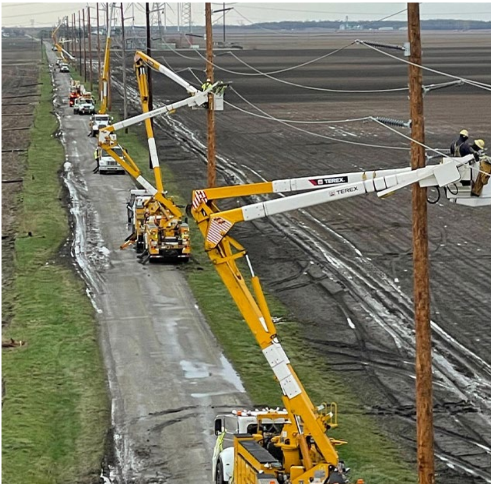
NIPSCO transmission repair work after storm damage in April | Northern Indiana Public Service Co.
