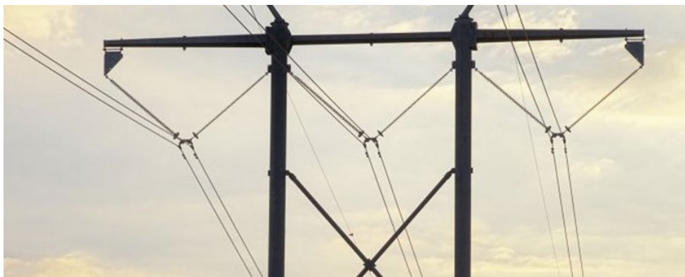
Republic completed the Duff-Coleman line in 2020 | LS Power
