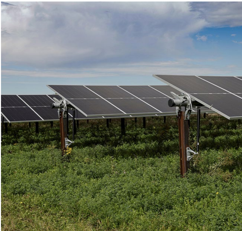
The Point Beach Solar Energy Center in Wisconsin | American Public Power Association
