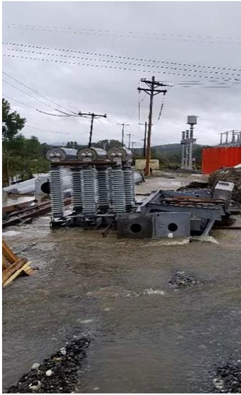
Flooding at the Adams #21 substation | National Grid
