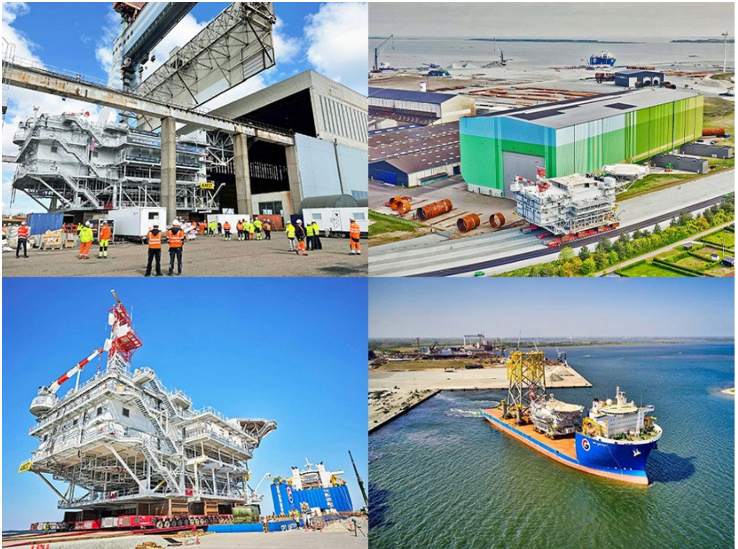
A 3,200-ton substation is moved out of the Bladt Industries factory in Denmark and onto a ship Thursday for transport to the Vineyard Wind 1 offshore wind project in Massachusetts. | Bladt Industries
