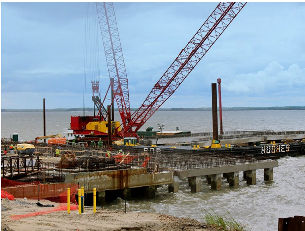
Construction of the New Jersey Wind Port on the bank of the Delaware River in South Jersey | © RTO Insider LLC
