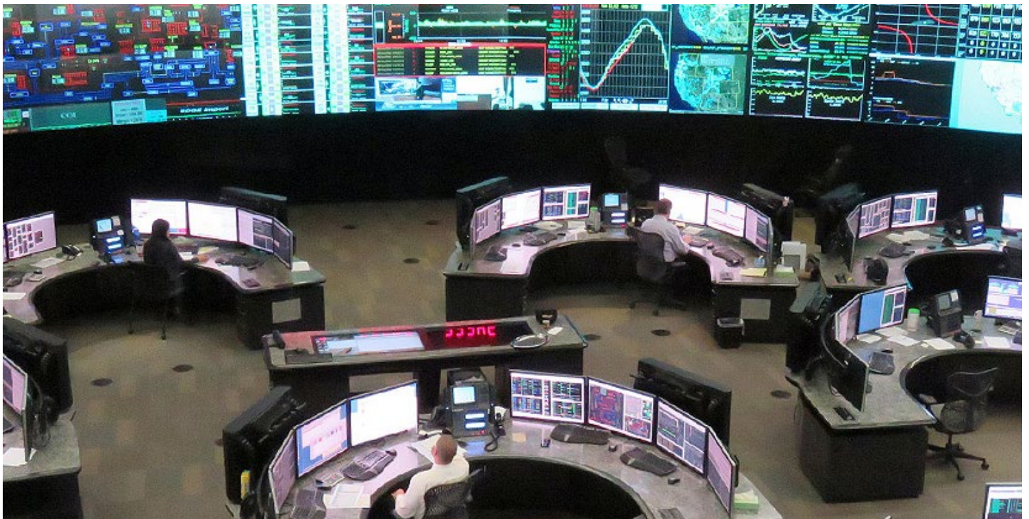
CAISO Control Room | © RTO Insider LLC
