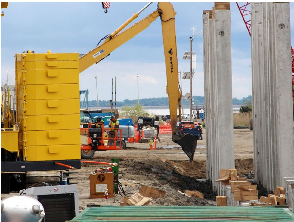
Workers prepare piles to be pounded into the ground at the New Jersey Wind Port in Lower Alloways Creek, South Jersey. | © RTO Insider LLC
