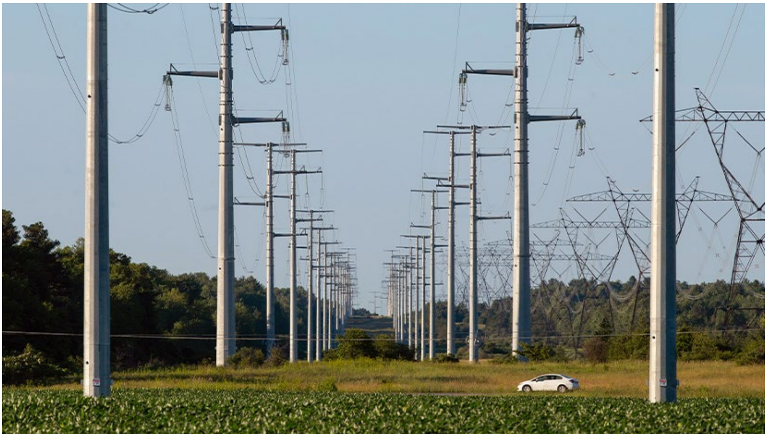
Modernized steel 345kV transmission Clean Path lines | NYPA
